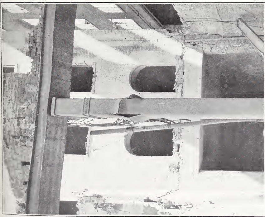
8. FAILURE OF CAST-IRON SHELL OF CONCRETE-FILLED CAST-IRON COLUMN BY FIRE, ACADEMY OF SCIENCES BUILDING, SAN FRANCISCO
